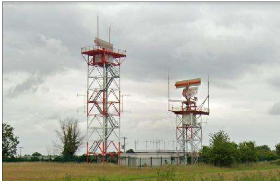
Figure 13. Dublin Airport MSSR Radar Station #2
